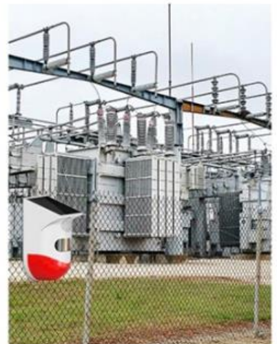
Power station area
